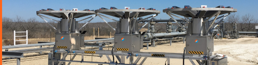
1500 watt Auto-CP system on natural gas pipeline, Texas, USA
